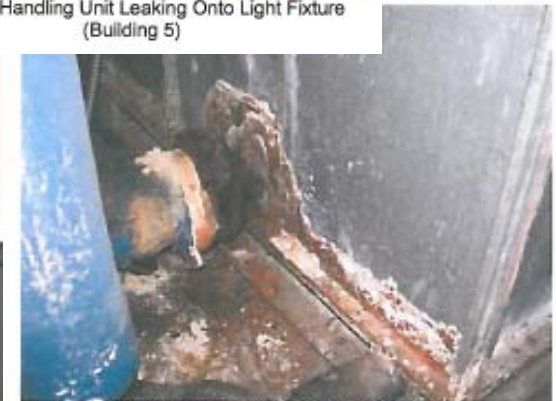
Multizone Unit Coil Casing Corrosion (Typical Buildings 1-4)
