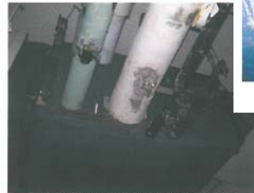
Shop Air Handling Unit Casing Corrosion (Typical Building 5)
