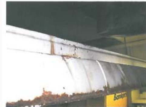
Shop Air Handling Unit Leaking Onto Light Fixture (Building 5)
